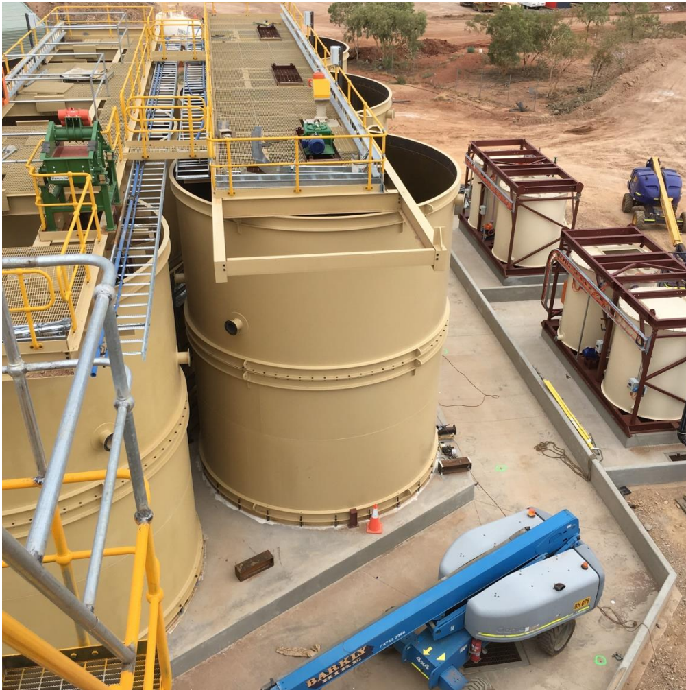
CIL Plant on site
