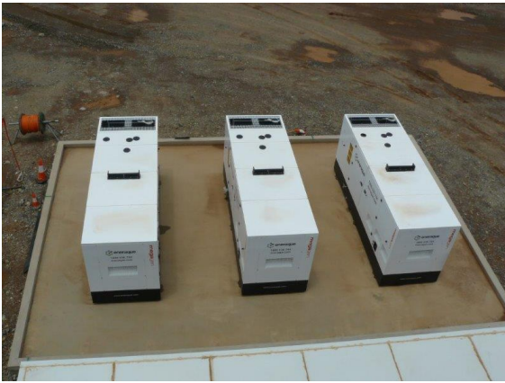
Generators on site
