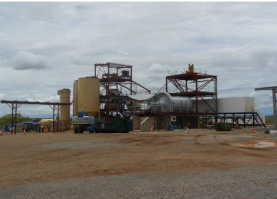
Process plant – equipment installed
